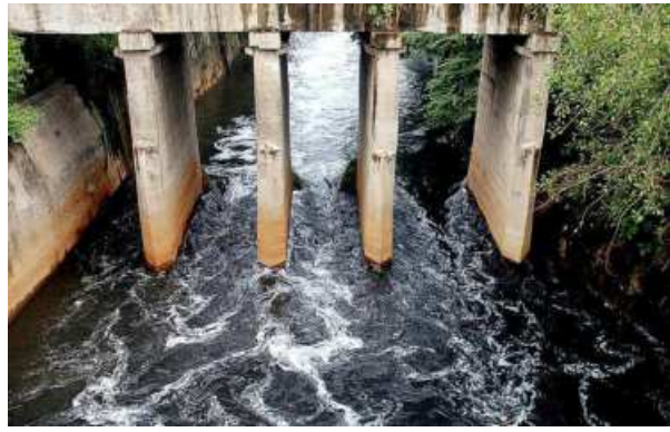
In need of rejuvenation: Najafgarh drain contributes about 40% of the pollution in the Yamuna. FILE PHOTO
